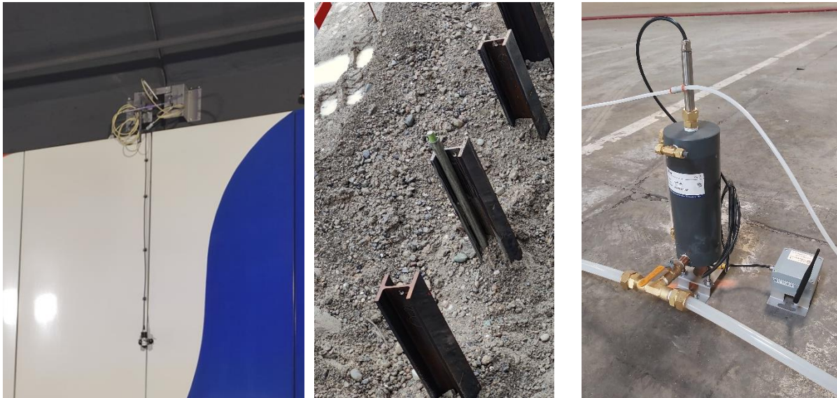
Figure 6 Examples of geotechnical sensors: 3D crack meter, In-place inclinometer and Hydrostatic levelling equipment
