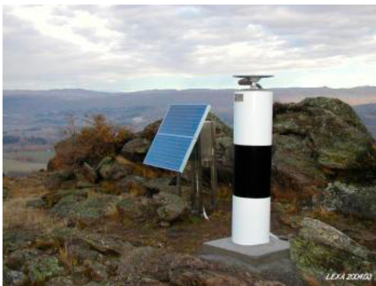
Figure 12: Example of a typical GNSS Continuously Operating Reference Station (CORS) installation.
